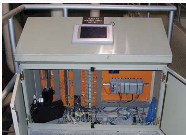
Filter control panel post-commissioning, in which, the new controller and HMI interface panel have replaced the legacy system highlighting a much “cleaner” installation.
