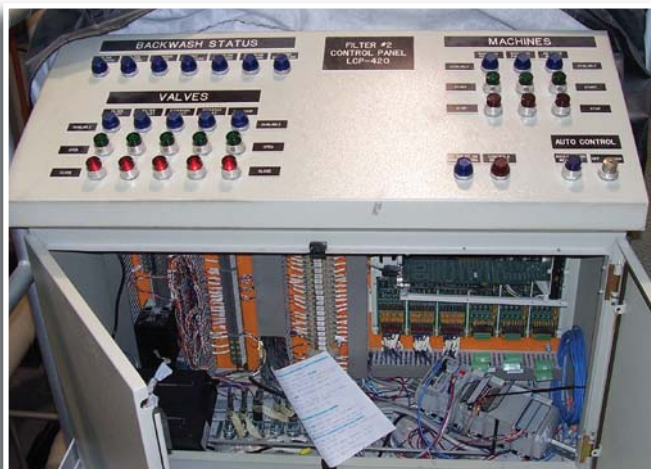
Filter control panel depicting the legacy and new PLC controllers on the same I/O set.
