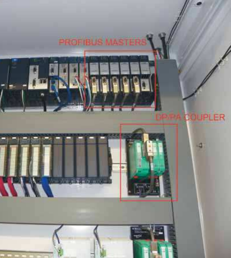
Figure 1: Fieldbus systems connect devices (sensors, actuators, flowmeters, etc.) to the PLC by means of a single control cable (bus) connected to a "master" module located in the PLC rack.
